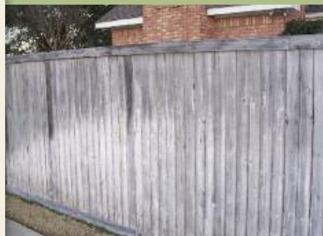
Almost 20 years after it was installed, this section from Mike Cork's fence still repels water.
